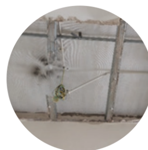
Collapsed False Ceiling
