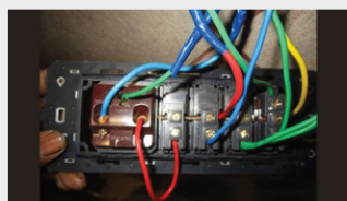
Naked wire used for switch to switch parallel connection
